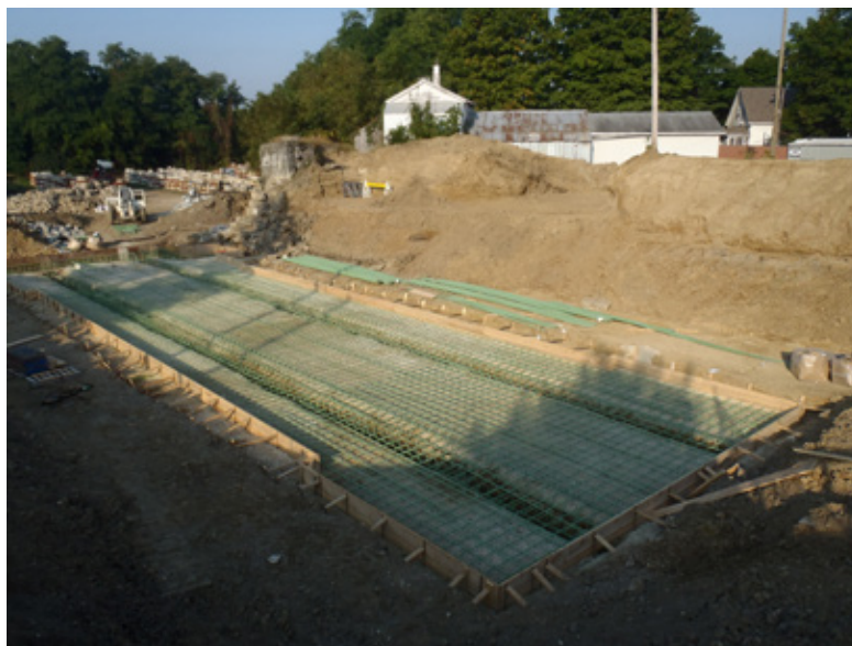
Forms for pouring concrete to create a strong foundation for rebuilding the lock.
