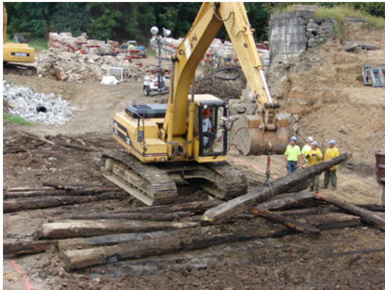
Removing oak timbers from original lock, with salvaged lock stones organized in the background.
