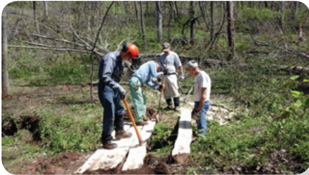
The Buckeye Trail Crew building a "new" short bridge at AEP ReCreation Lands.
