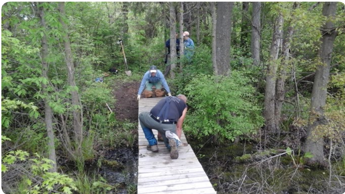
Replacing one of the bridges near Junction across the canal (photo by Richard Lutz)
