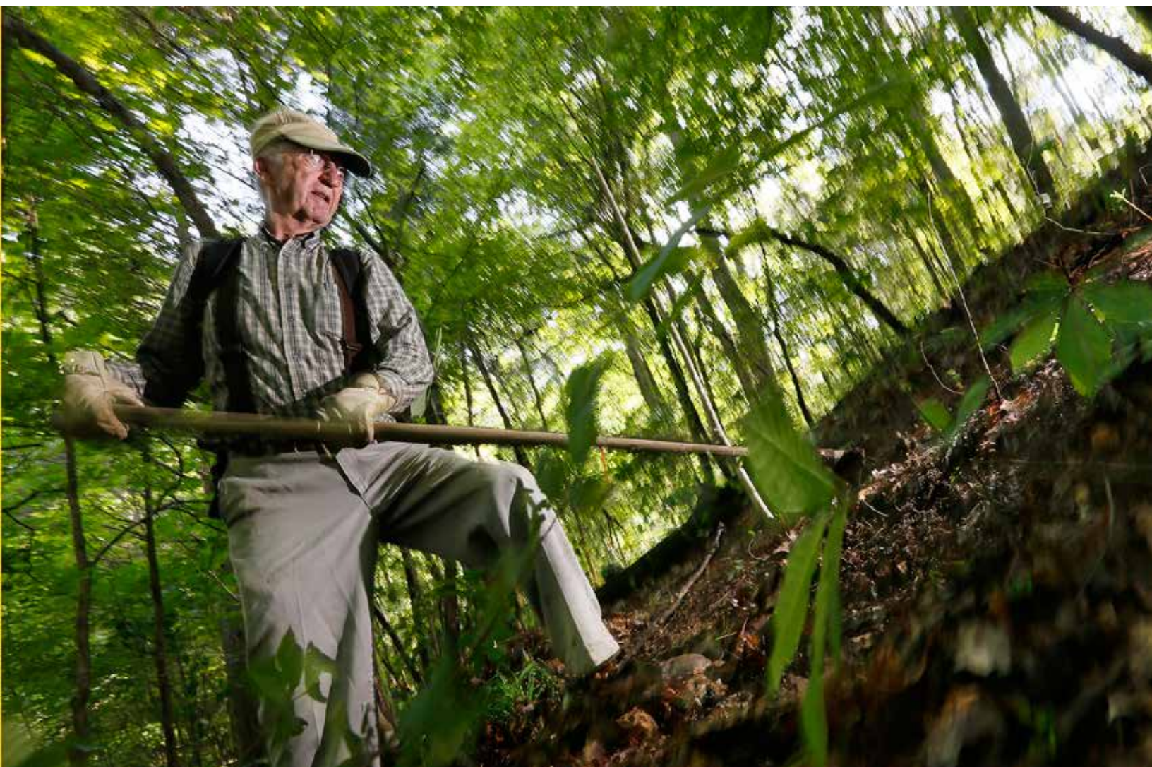
Elmo Layman building new BT at the Nature Conservancy Edge of Appalachia Preserve.
