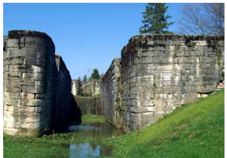
Example of a lock in need of repair (Lockington Locks)
